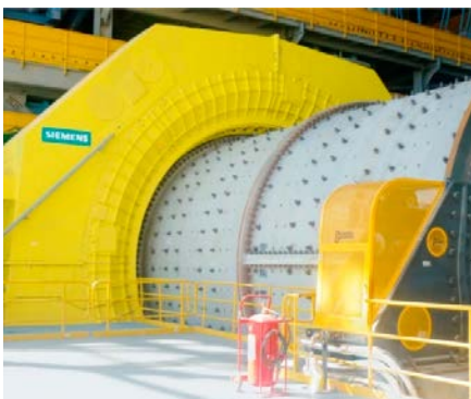
Capacitive sensors are also used for air gap measurement in large electric motors.
